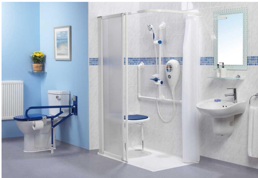
Photo Credit: PFM -Accessible shower room for domestic use (https://www.pfmuk.org/wet-room/)
